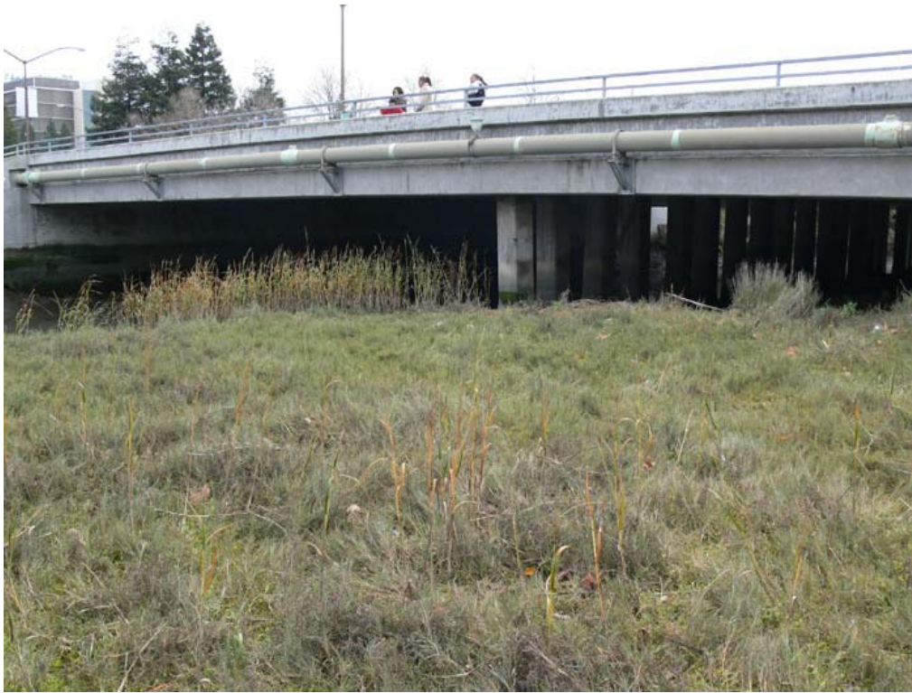
Photo 1 - View of Veterans Blvd bridge over Redwood Creek; pickleweed and cordgrass in the foreground
