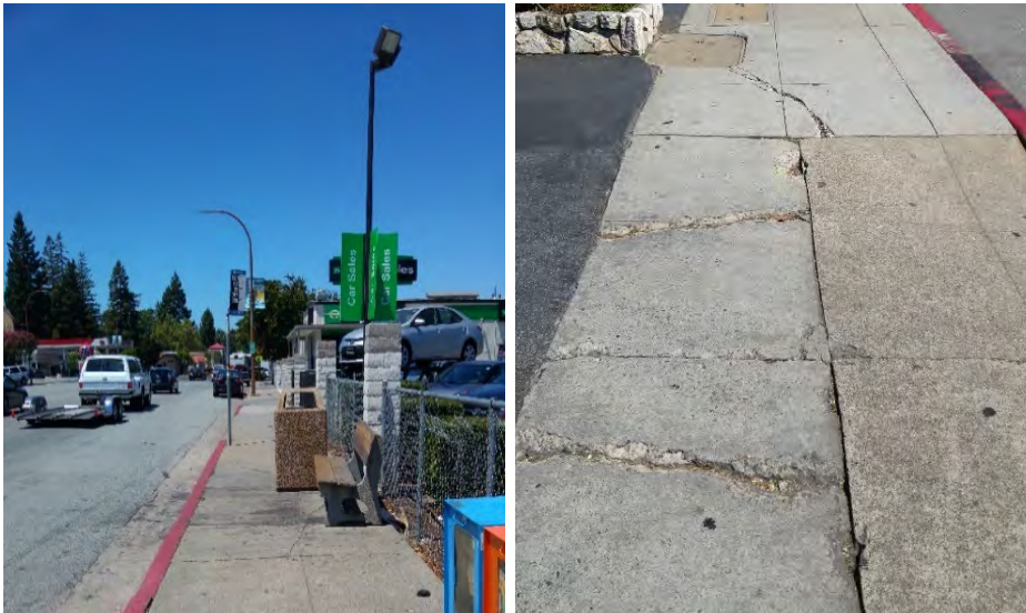
Street furniture on narrow sidewalks (left) and cracking on existing sidewalks (right).
