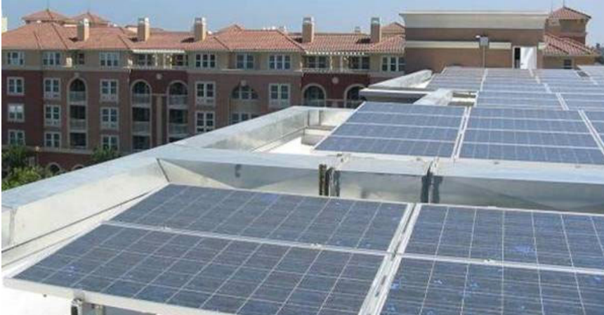
Solar panels located on the Villa Montgomery residential apartment building on El Camino Real
