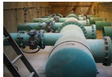
Water pipes in Redwood City
