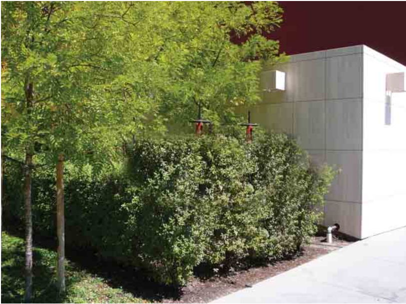
Utilities and equipment shall be screened from view by landscaping, screen walls, and/or equipment enclosures painted to blend with the landscape.
